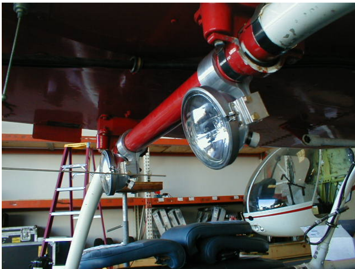
G3-1 Landing Light Installation
